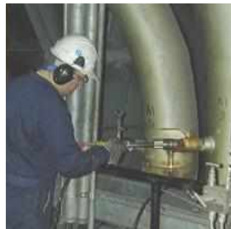
ASME PTC 4.2 sampling in a coal pipe
