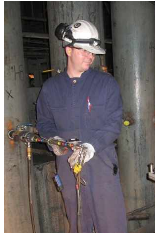
Velocity testing in a coal piping system
