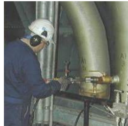
ISO 9931 sampling in a coal piping system
