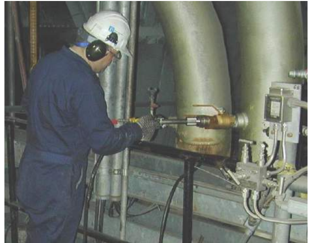
IsoAsh sampling in a piping system
