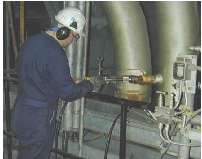
IsoAsh sampling in a piping system
