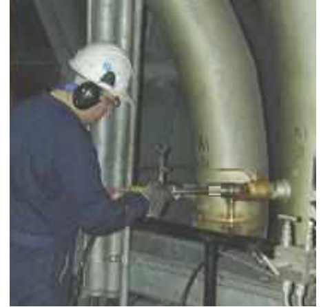
ISO 9931 sampling in a coal piping system
